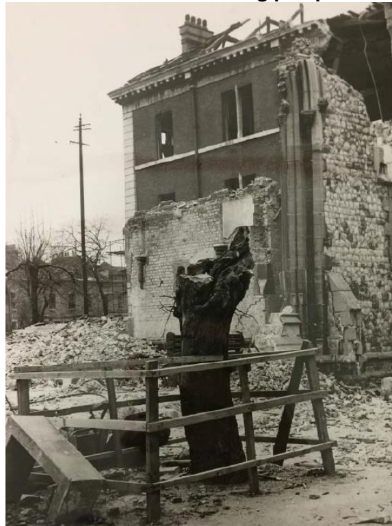
Figure 33: Bomb damage to the Mulberry Tree with the bomb damaged Chapel and North Wing to the rear.
